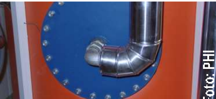
Not like this: uninsulated storage tank connections
