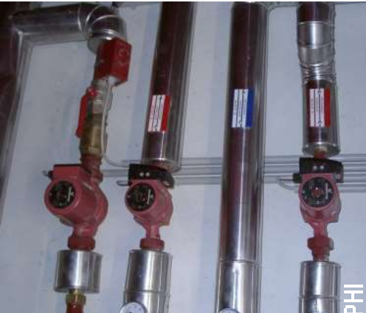
Not like this: uninsulated pumps
